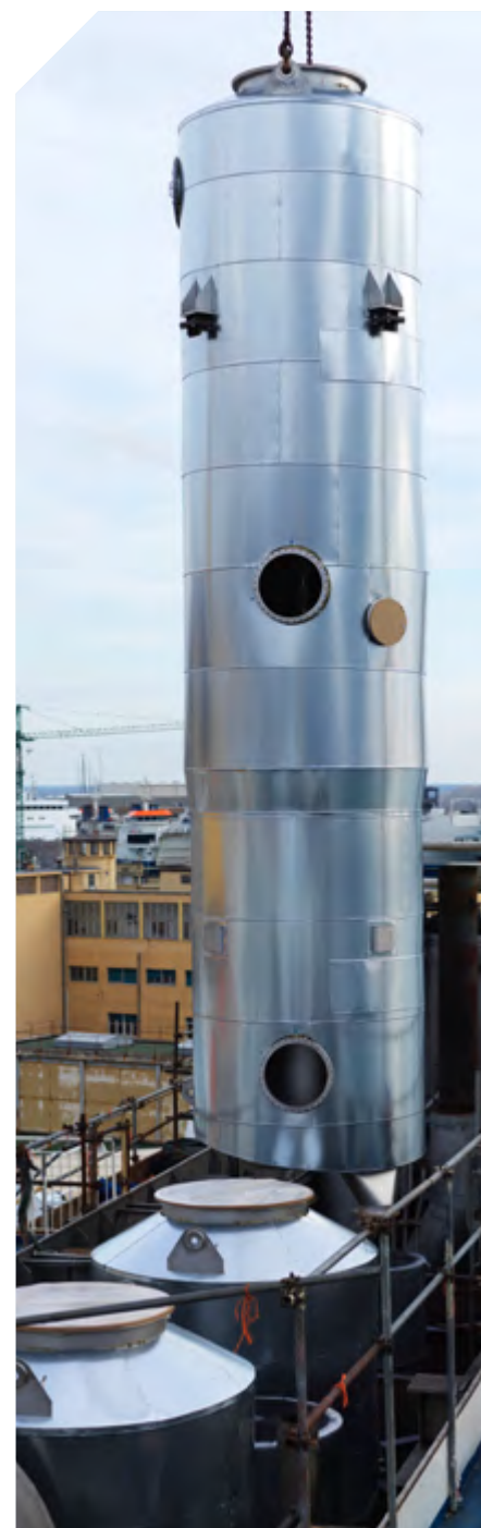
An Ecospray scrubber is installed
